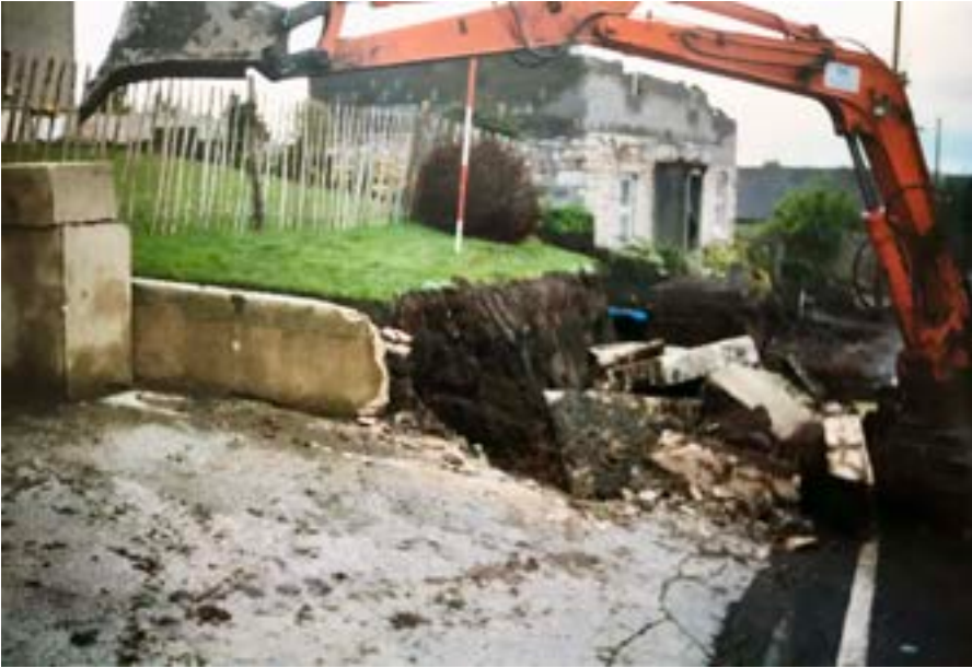
Road widening in progress during the 1980s. The cottage being renovated was 'Homleigh', possibly dating back to at least 1724 when it was known as 'Stockwell Farm'. Courtesy of Joan Belt.
